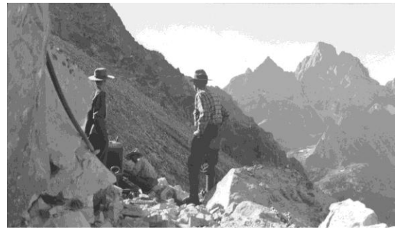
Figure 2. Trail construction often employed a compressor and drills used to fracture rocks or to prepare for blasting. This equipment was heavy, yet small compressors were conveyed far up the trail.
